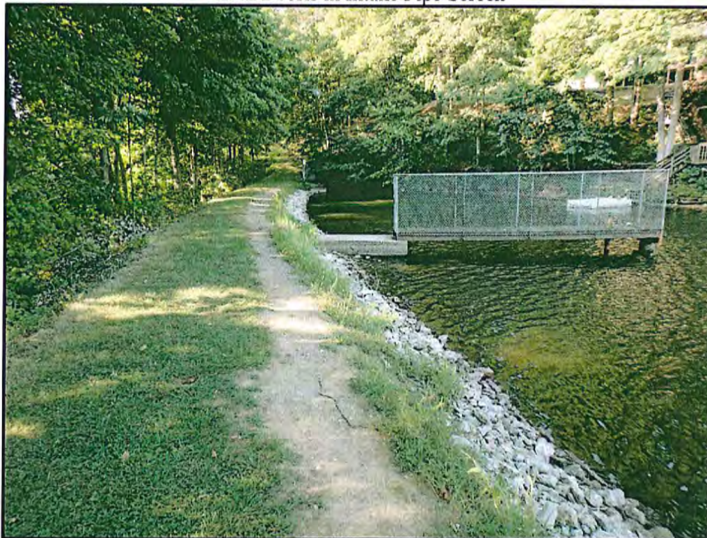
Photo 4: Gate Valve Platform for Outlet Works
