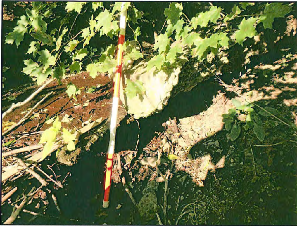
Photo 9: Principal Spillway Channel – Note Undermining of Left Training Wall
