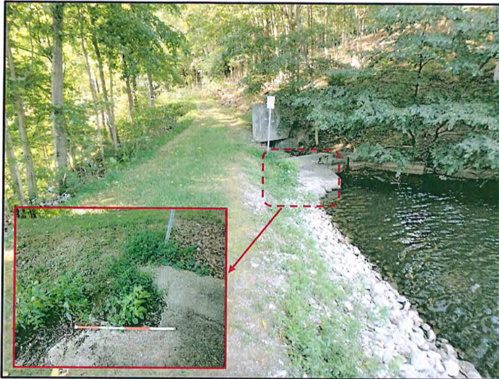
Photo 5: Principal Spillway Weir – Note Void in Concrete (See Inset)
