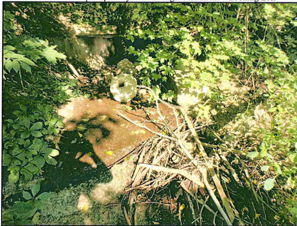
Photo 8: Principal Spillway Channel – Looking Upstream; Note Debris and Concrete Deterioration
