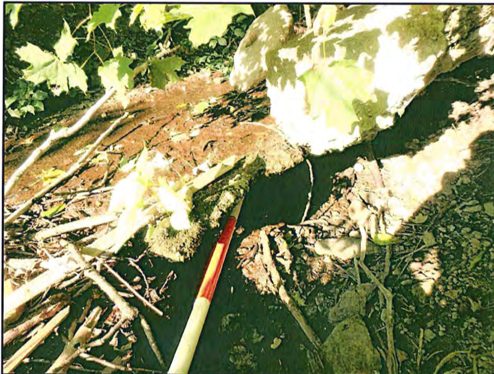
Photo 10: Principal Spillway Channel – Note Undermining of Spillway Slab
