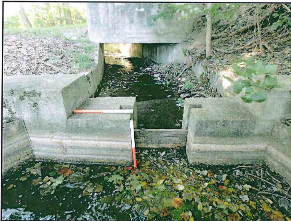
Photo 6: Principal Spillway Weir – Note Debris in Spillway Channel
