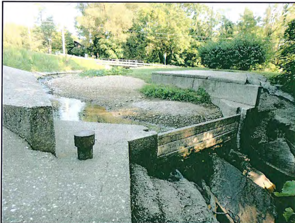
Photo 2: Intake Structure – Note Concrete Deterioration and Leakage Past Wooden Stoplogs
