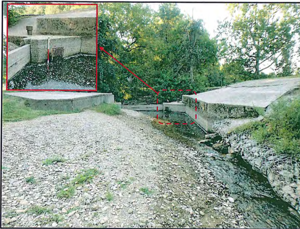
Photo 3: Intake Structure – Note Sediment Accumulation and Leaf Debris in Intake Pipe Screen
